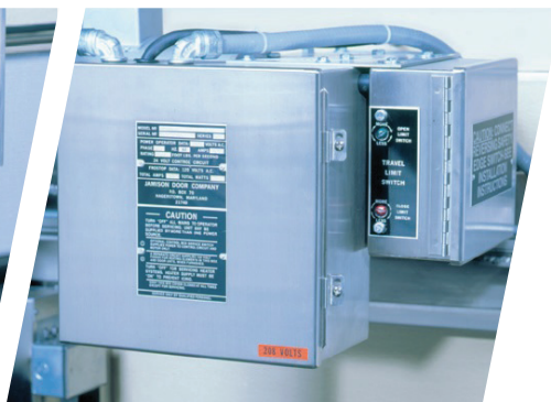
NEMA 4X Control Panel
